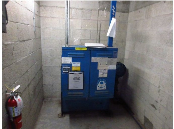
VIEW OF ELEVATOR EQUIPMENT
