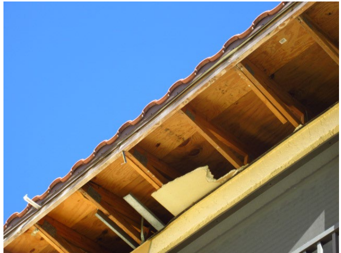
VIEW OF DAMAGED STUCCO
