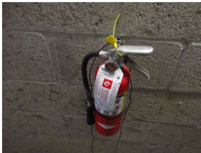
VIEW OF TYPICAL FIRE EXTINGUISHER
