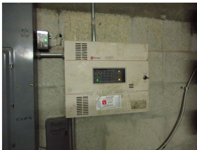
VIEW OF CENTRAL ALARM PANEL
