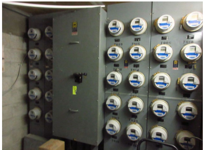
VIEW OF ELECTRICAL EQUIPMENT
