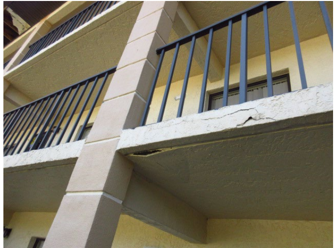
VIEW OF DAMAGED STUCCO
