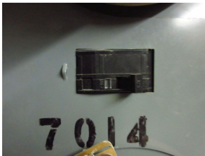
VIEW OF ELECTRICAL EQUIPMENT
