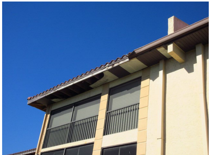
VIEW OF DAMAGED STUCCO
